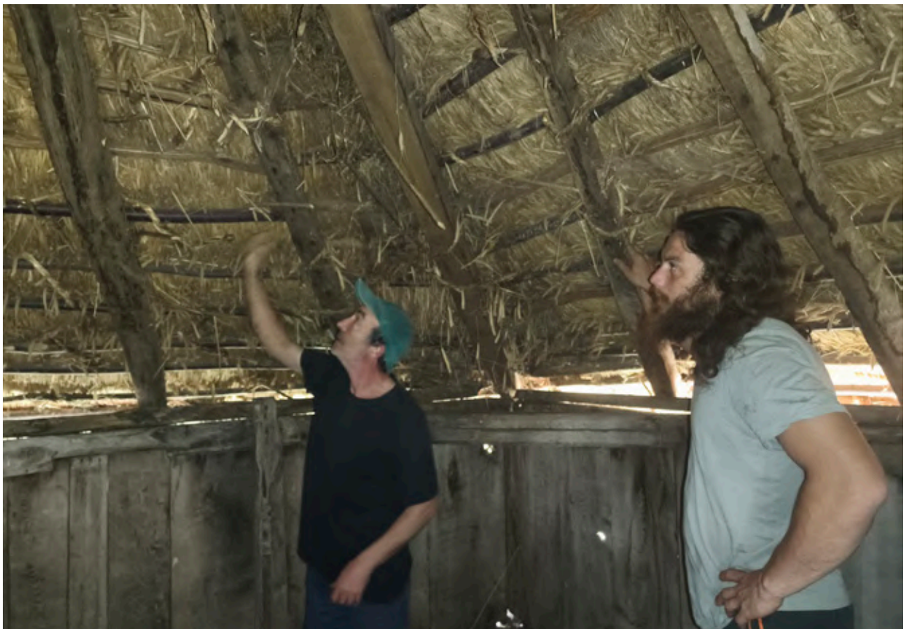
Condition assessment of a techo prior to intervention
